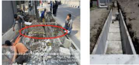
Figure 2. Subgrade Conditions with Uneven Compaction
