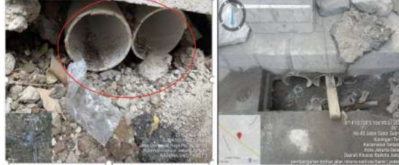
Figure 5. Initial Sedimentation Due to Lack of Work Area Protection
