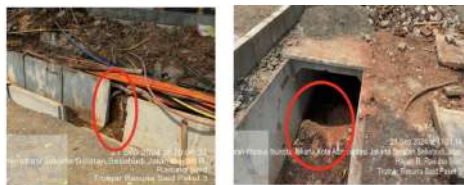
Figure 4. Initial Sedimentation Due to Lack of Work Area Protection
