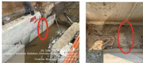
Figure 3. Channel Connection that is not Completely Closed
